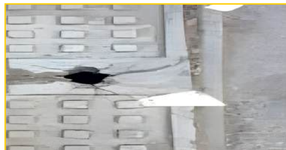
Condition of the Regular keyhole lifting arrangement of other make FRP manhole covers.
